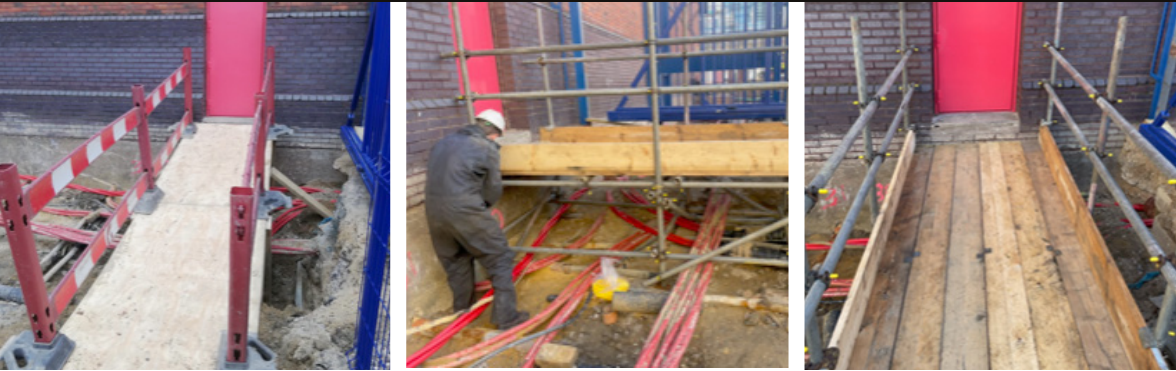
Provision of temporary access at Simpson Road Substation by erecting a small bridge over a freshly dug cable bay.
